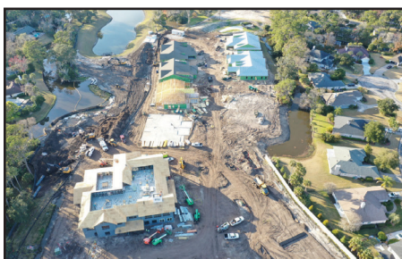
Eight of the 43 proposed cottages, which will be duplexes and triplexes, are currently under construction with the first ones set to be finished in March and all of them completed by early November.
