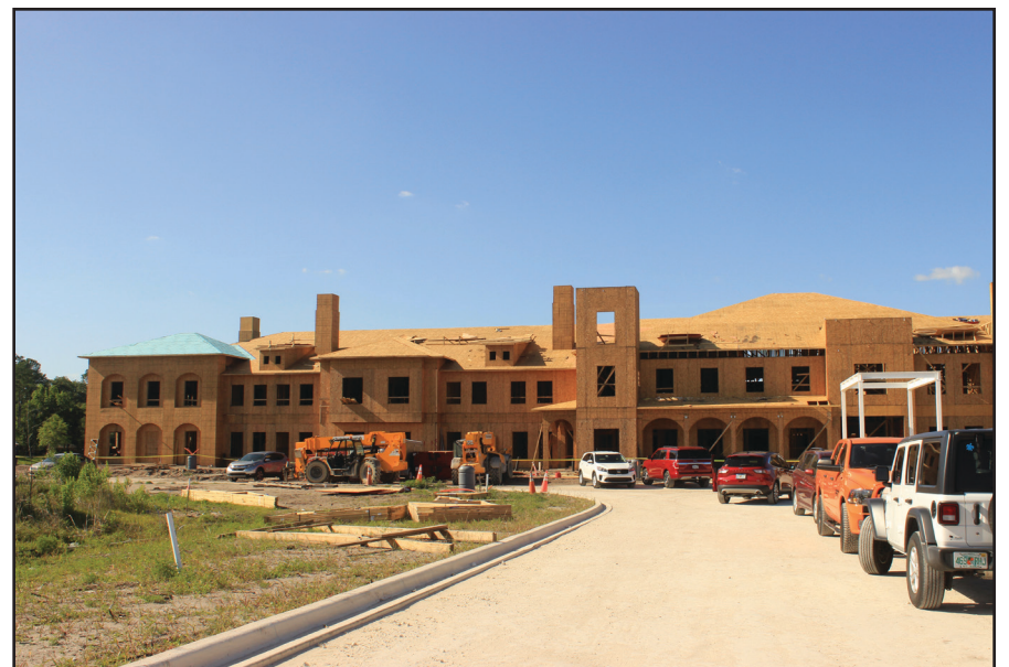
The Blake at St. Johns is under construction. It will be located at 2430 County Road 210.
