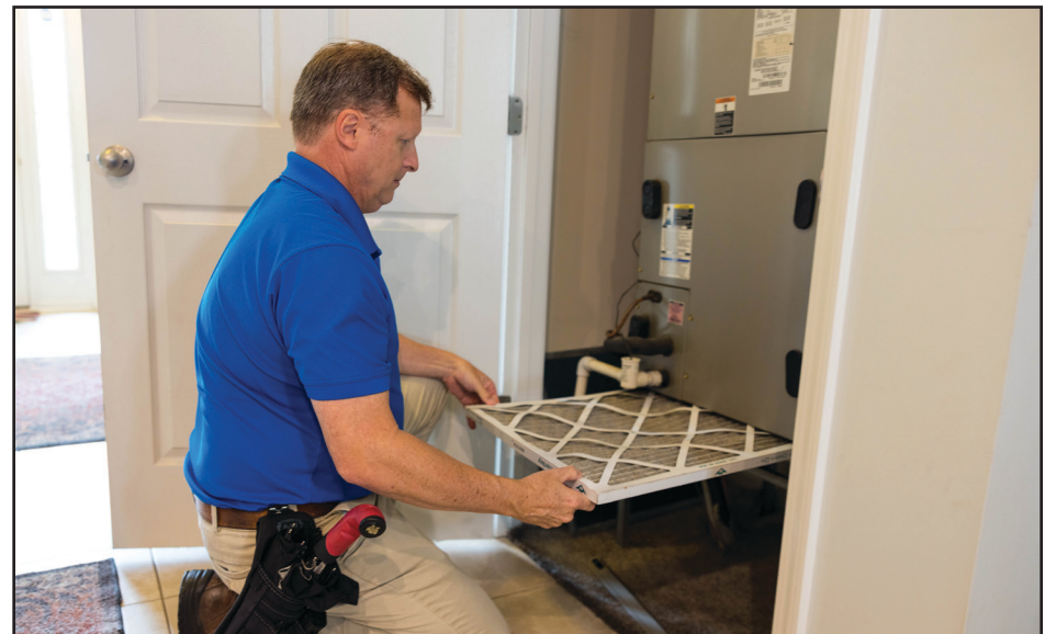
Mock also recommends changing air filters regularly.
