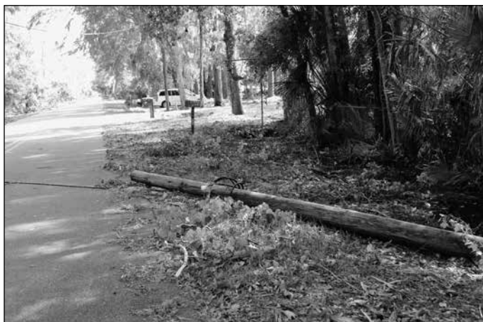
Power lines were down across Ponte Vedra and the Beaches in the aftermath of Hurricane Matthew.
